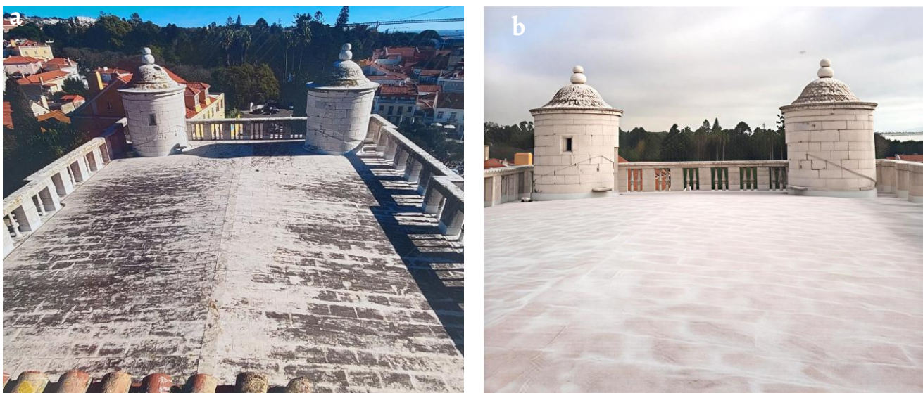
Figure 9. Chancel's roof: a) before (photos: Nova Conservação, S.A.) and b) after the intervention, 2023.
