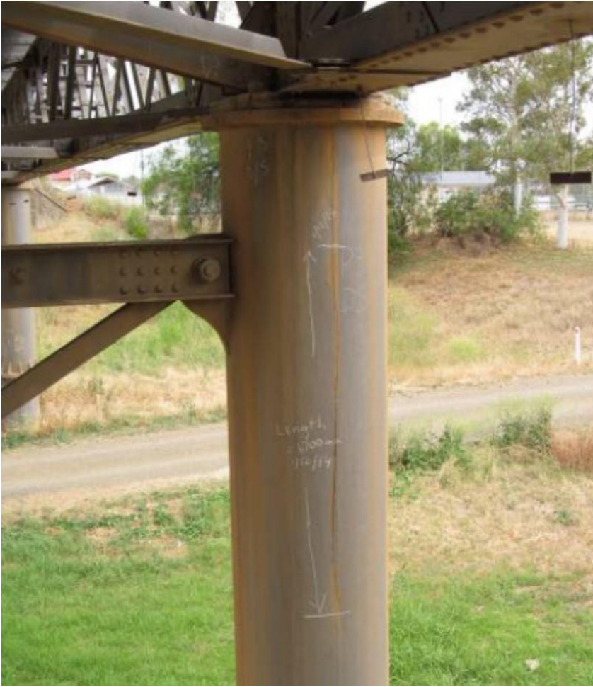
Figure 4. Crack in Pier 3 column (photo: C. Everett, 2017).
