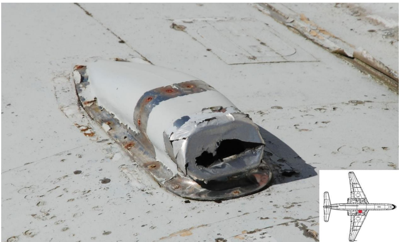
Figure 5. Failed bitumen based flashing tape from the 1990s.
