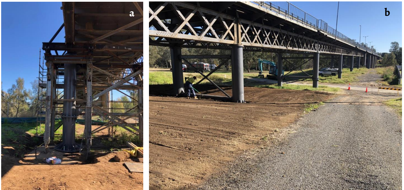
Figure 8. Bridge: a) completed column; b) new piers in place (photos: A. Rosnell, 2021).
