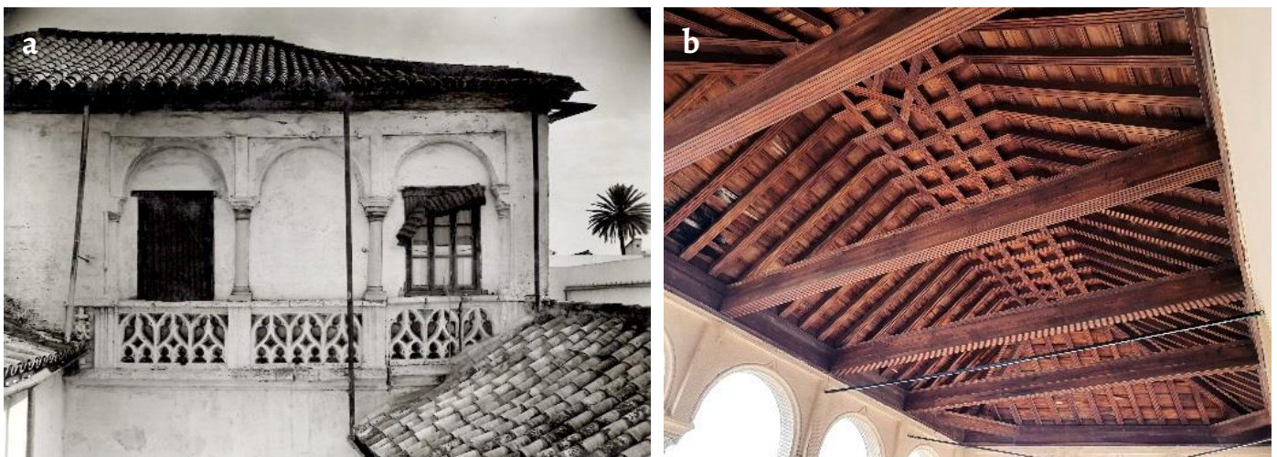
Figure 5. Lookout-tower of the Pensión Don Marcos: a) prior state towards 1950 [23]; b) reconstructed frame. Authors' photography (2021).
