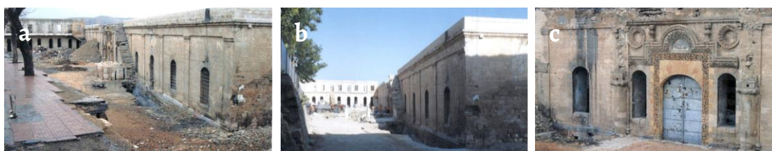
Figure 5. Views showing the status of the building, which remained empty, photographs by Şanlıurfa Regional Board of Conservation of Cultural Heritage.
