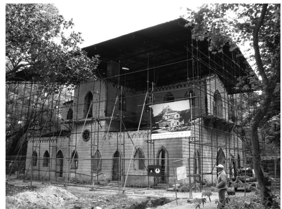
Fig. 2 Current condition after the fire in 1999 (September 2007).
