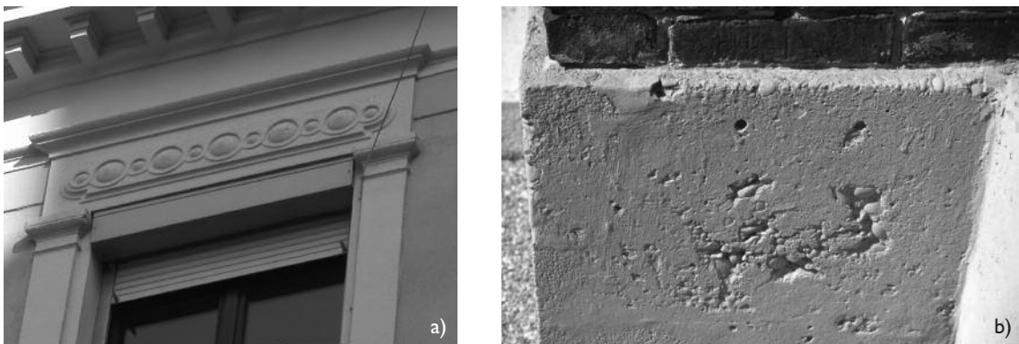
Fig. 3 A yellowish or brownish painting is generally applied on the ancient concrete, with (a) or without (b) preliminary application of a Portland-cement-based surfacing mortar.
