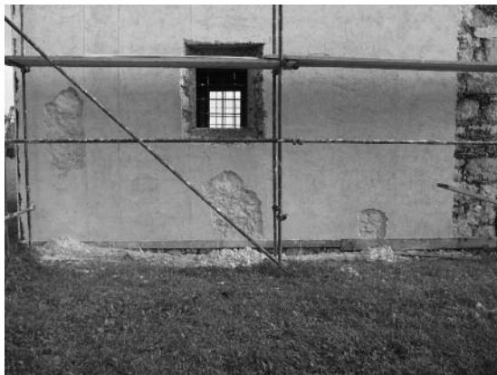
Fig. 5 Thicker parts of rendering layers were falling from the wall after rain.
