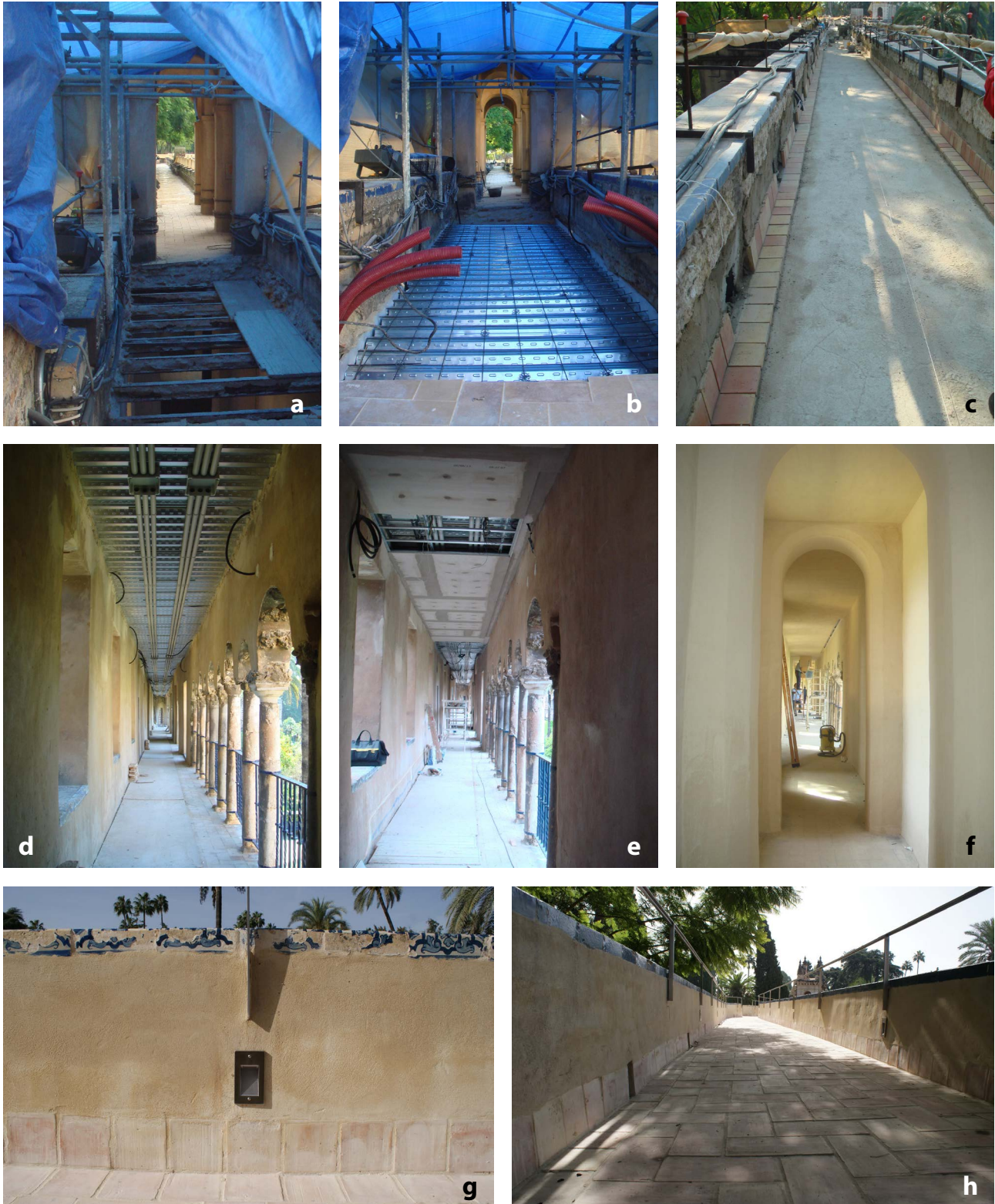
Figure 6. a) Demolition. b) New roof deck profile. c) Beginning with the handmade ceramic floor tiles. d) Installations under the roof deck profile. e) False ceiling. f) Interior final state. g) Small lamps connected to a double circuit to provide normal lighting and emergency lighting. h) Final state of the walkway.
