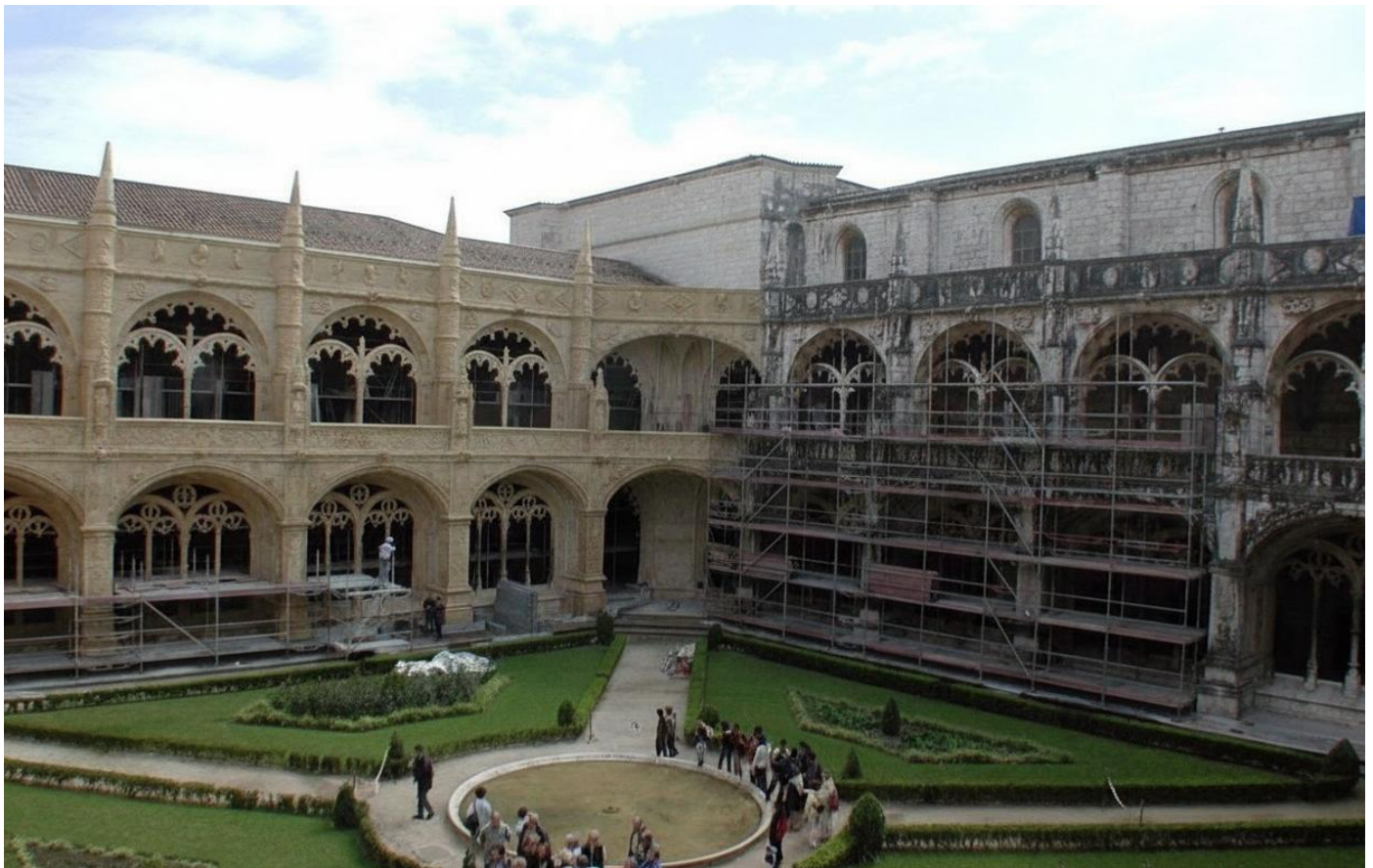
Figure 5. Ongoing works in the cloister, with visitors contemplating the intervention, c. 2000 (photo: D. Caldeira).
