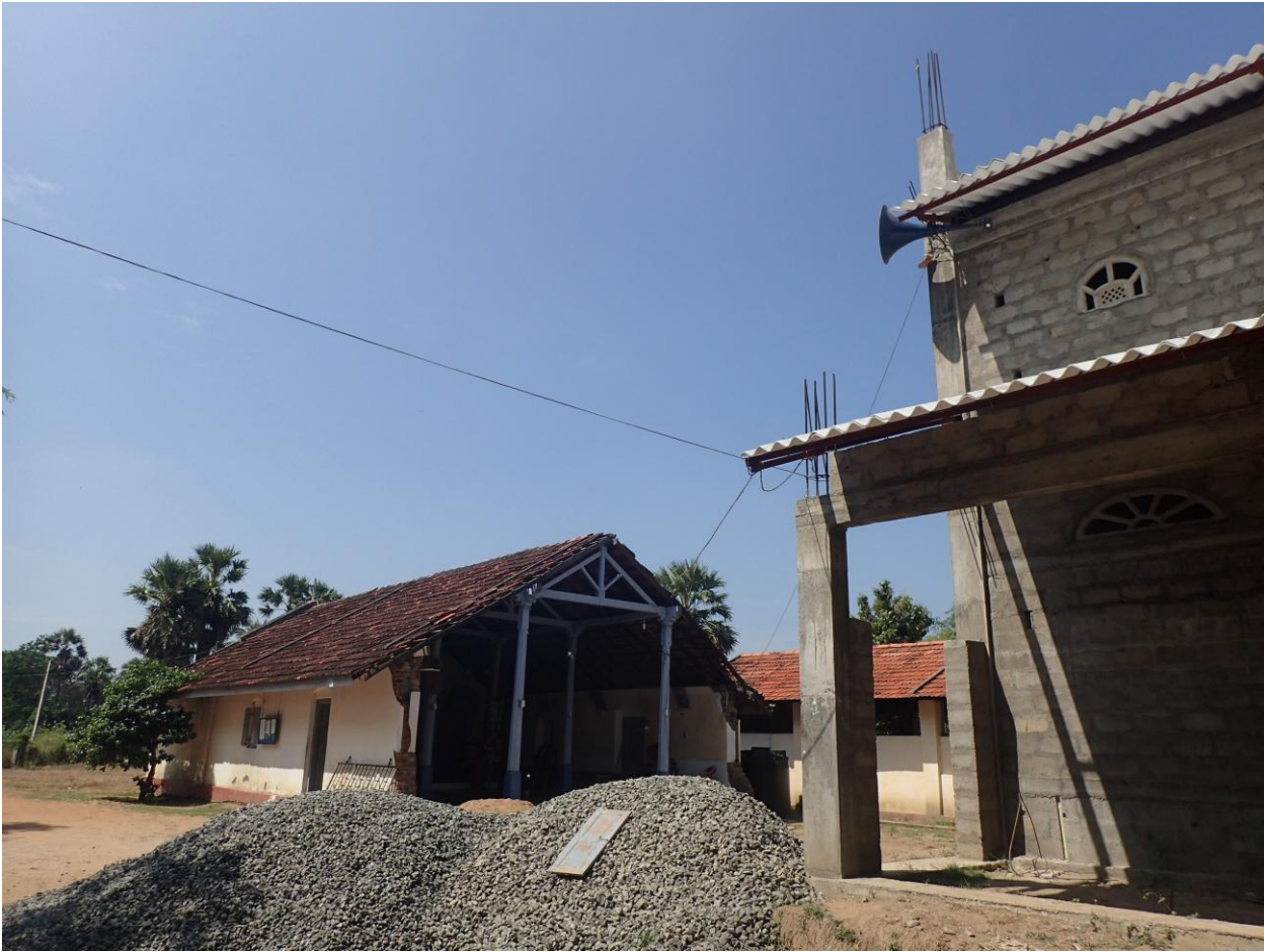
Figure 3. Holy Rosary Church in Palayadipudikulam, Mannar, in 2018 during its demolition, while the new church was being constructed in front of it (photo: Joaquim Rodrigues dos Santos).
