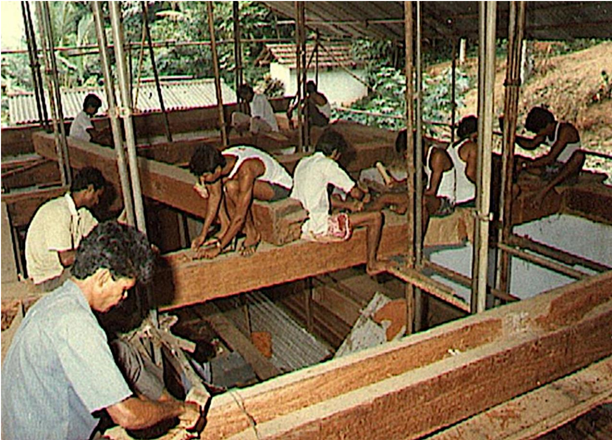
Figure 11. Restoration works on a historic monastic building, famous for its wooden architecture, in the 'Mahavihara' Buddhist Monastery in Kandy (photo: Jayatissa Herath).
