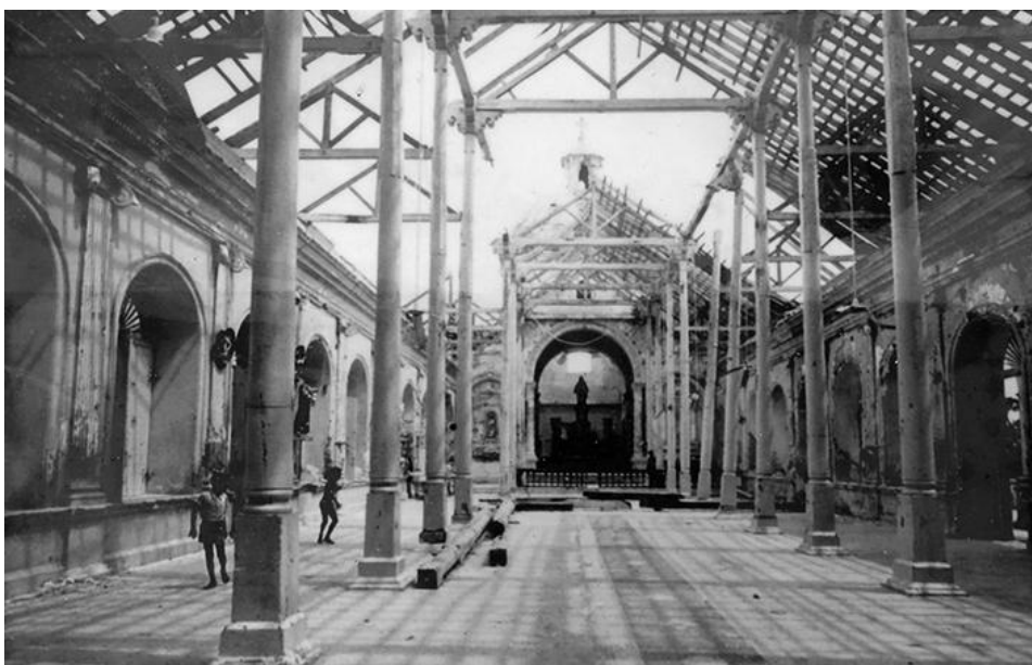
Figure 2. Inside of St James’ Church in Gurunagar, Jaffna, in 1993 after the aerial bombing during the civil war (1983-2009) (source: courtesy of the Parish Priest, St James’ Church in Gurunagar).
