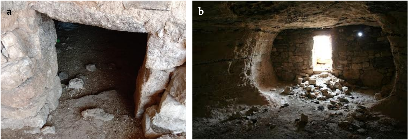
Figure 8. Abandoned and misused hermit caves that surround Machaerus Fortress, 2022: a) an interior view revealing stone collapse and physical deterioration; b) a cave interior demonstrating accumulated debris, lack of conservation, and ongoing neglect.
