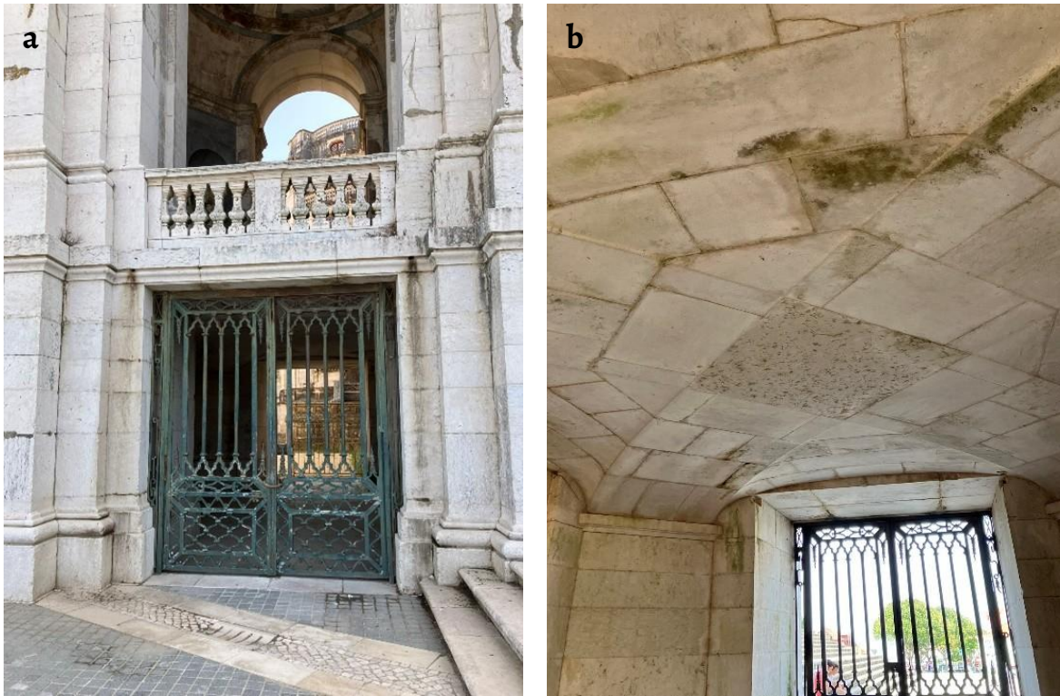
Figure 1. Vault: a) location of the vault in front facade; b) bottom view under the vault.
