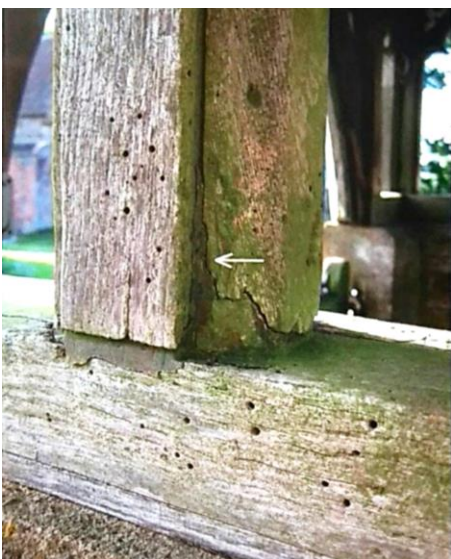
Figure 3. The white arrow points out the location of crack which indicates that the bond between resin and the decaying end grain of the timber was not strong, failure because of poor design [2, p. 318].
