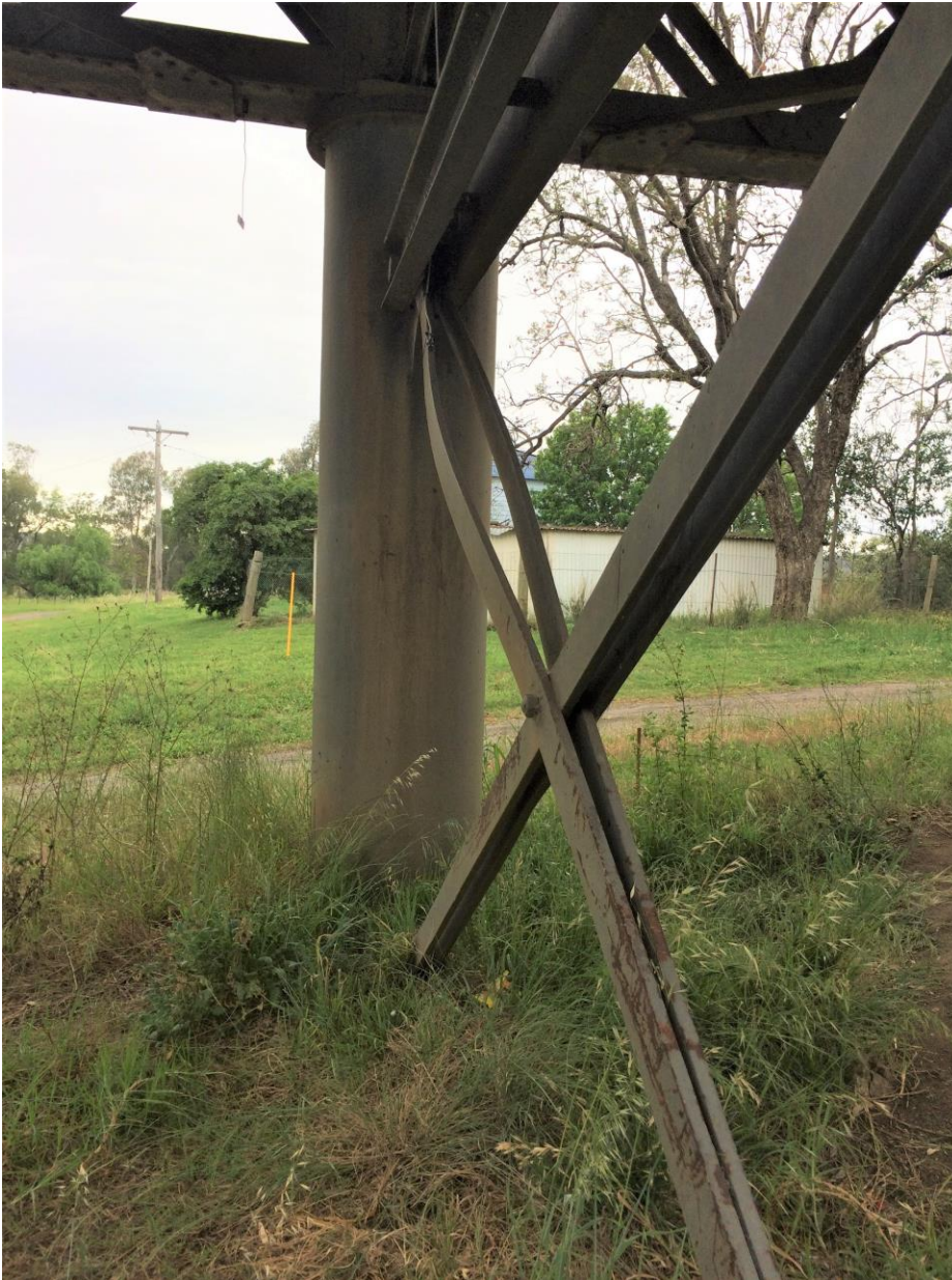
Figure 3. Buckled metal brace, Pier 1 (photo: C. Everett, 2017).
