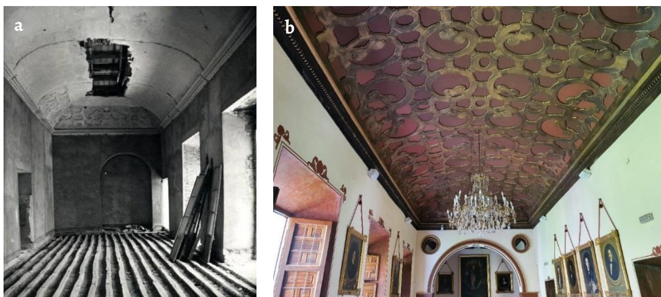
Figure 12. Plaster vault ceiling at the top floor main hall: a ) Prior state (1975) [24]; b ) Restored ceiling at the top floor hall. Authors' photography (2021).
