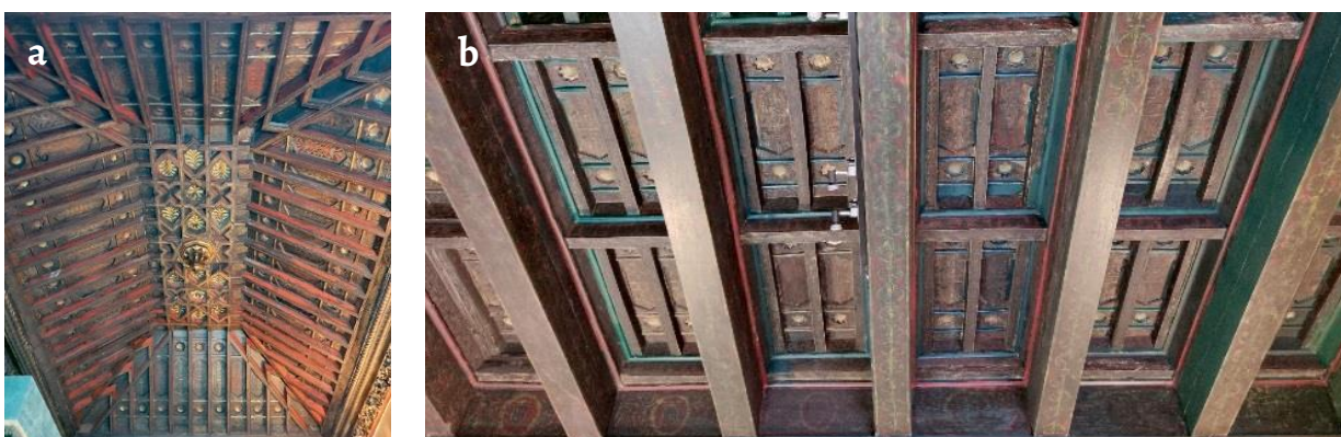
Figure 14. Ceilings: a) chapel's original coffered ceiling; b) coffered ceiling transferred to the antechapel. Authors' photographs (2021).
